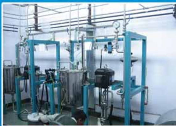
Paint Supply System - Pneumatic
